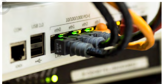
Figure 10.12: Cables connected to a network switch
